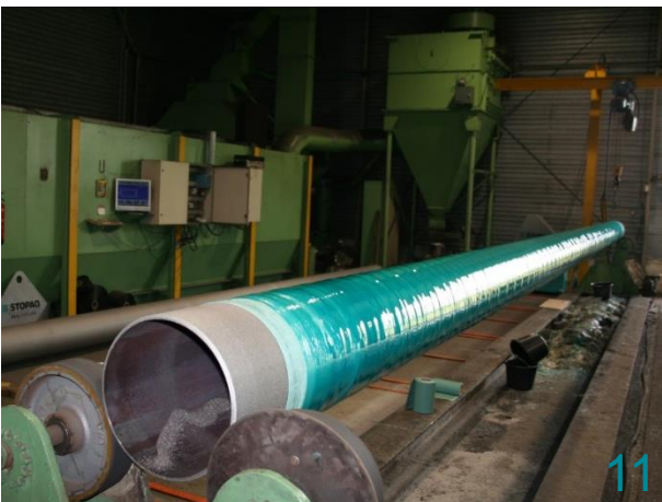
Immediately after finishing the physical application, start rotation of the pipe to avoid sagging of the uncured epoxy.
