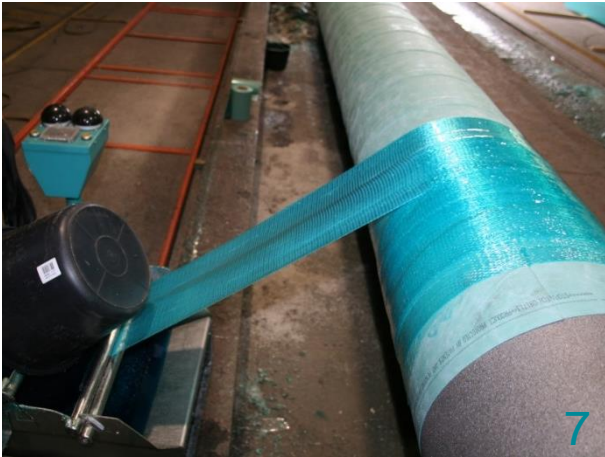
Remove the non-impregnated part of the FAST GRE Fabric and start wrapping. Overlap according to project requirements.
