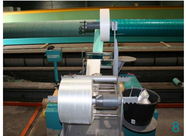
Depending on pipeline diameter, the angle of the FAST GRE Wrapping Device must be adjusted to ensure the needed overlap.
