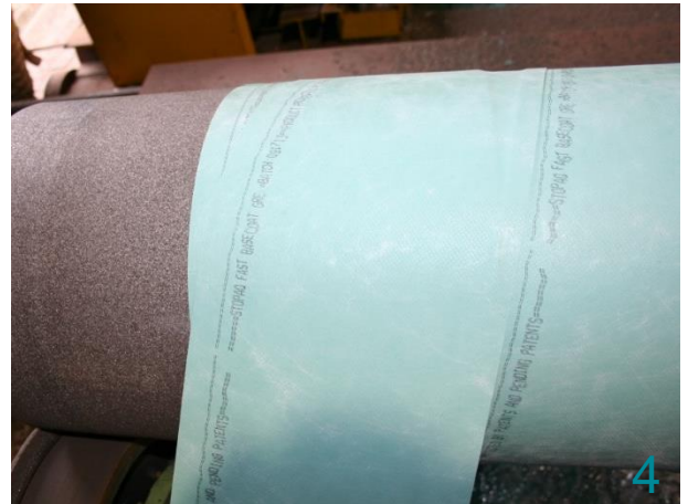
4 Continue until overlapping on the straight wrap FAST Basecoat and the entire area has been achieved. Conduct holiday test at 10kV with a brush probe.
