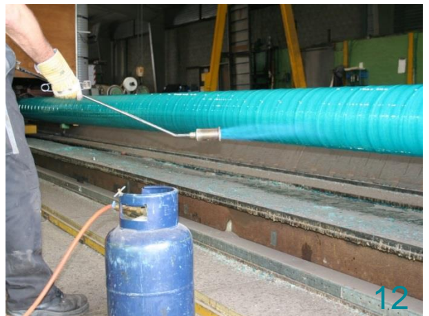
To ensure a smooth finish of the surface flaming of the surface of the applied coating system might be considered. This can be carried out by means of a propane gas torch just before pipe handling to the curing station (force cure).
