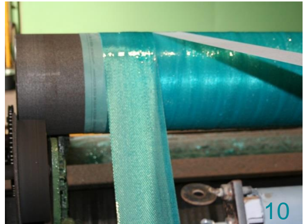
The FAST GRE Wrapping Device shall be placed perpendicular to the pipe before the final wraps are applied. Number of layers as per specification.
